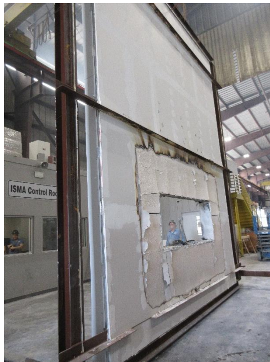
Photo No. 16 Damage Extent of Interior Sheathing – (Post-Mortem Observations)
