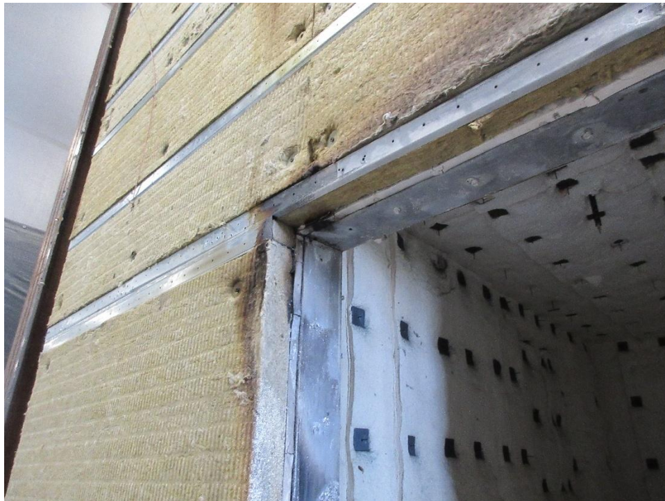
Photo No. 20 Damage Extent at Window header – (Post-Mortem Observations)
