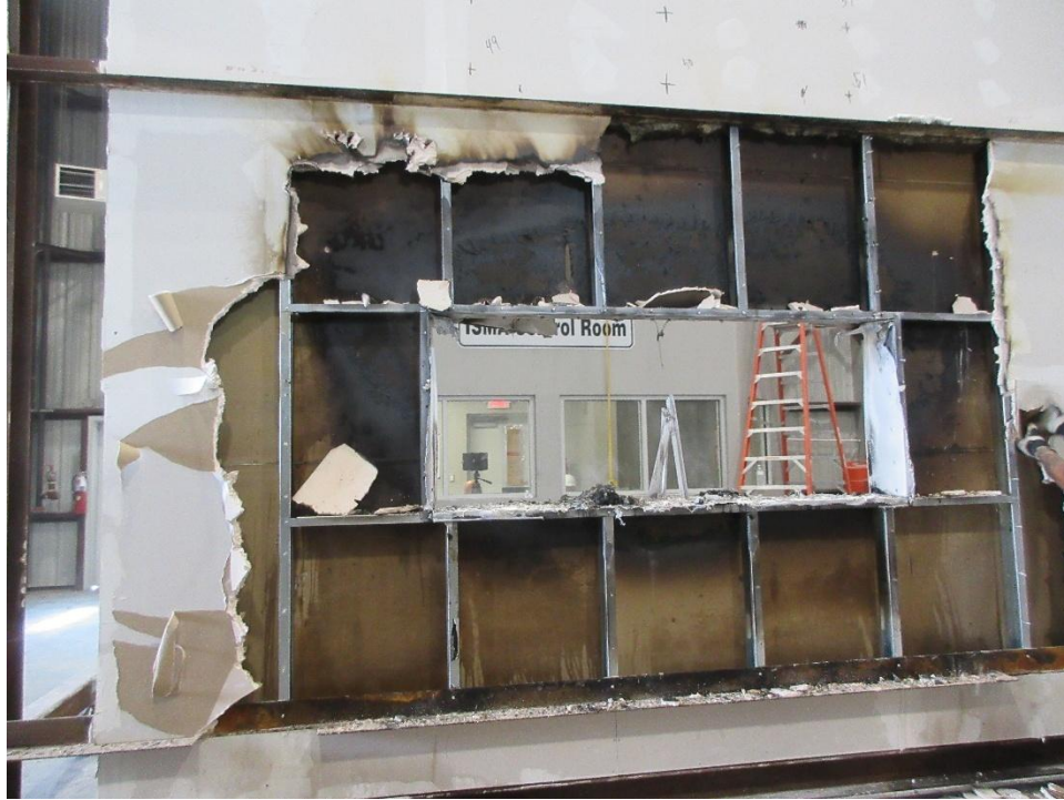
Photo No. 17 Damage Extent to backside of Exterior Sheathing – (Post-Mortem Observations)
